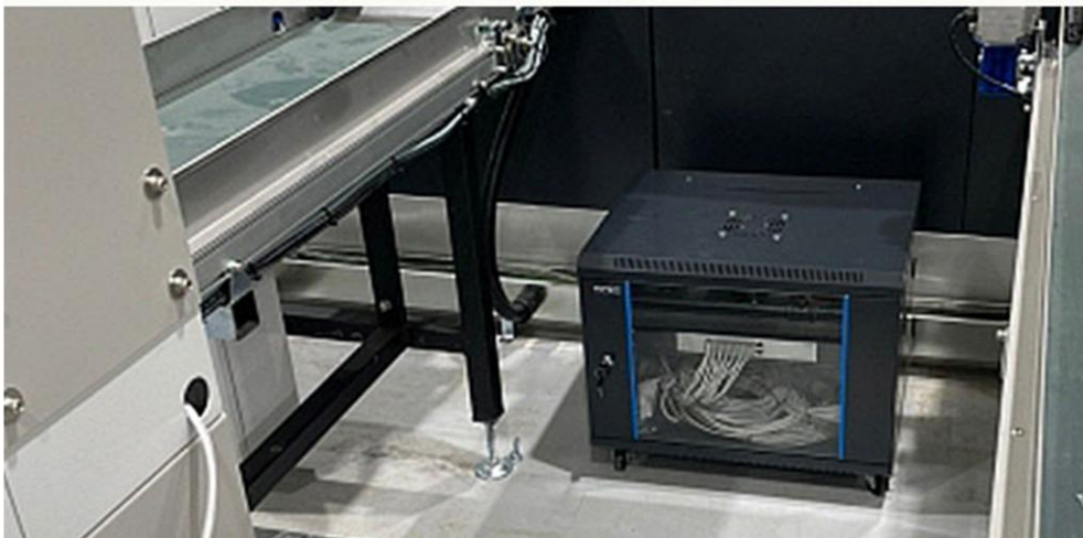
On-site Data Acquisition Hub
